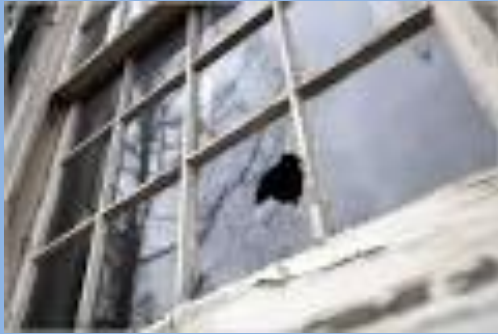
A single broken window, not repaired ...
