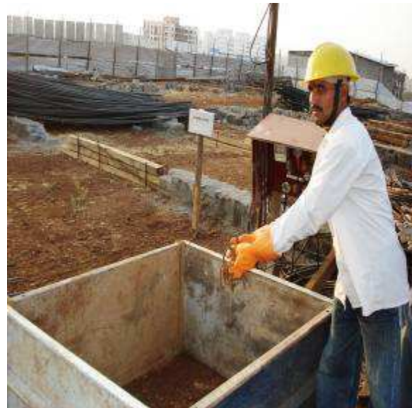
Safety violators accumulating the steel scrap & ring in a separate container
