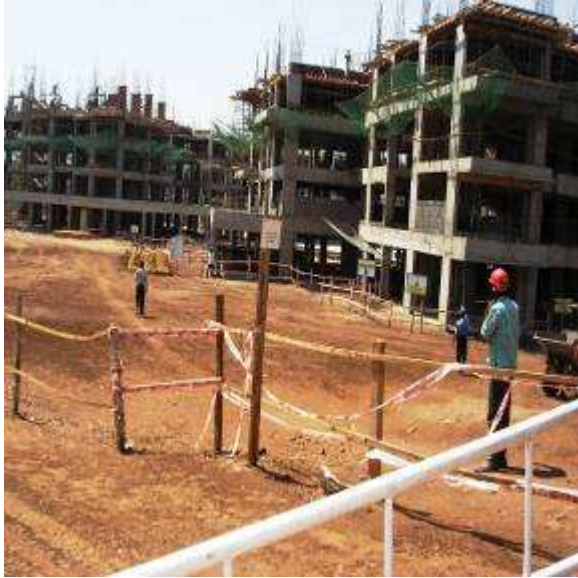
Security starting the sounding of alarm (whistle) inside the building
