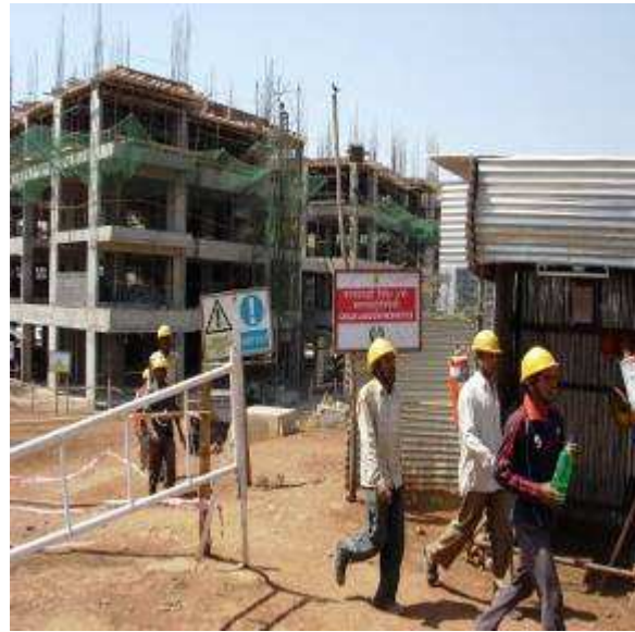
Remaining few workers coming out of the building & gathering at safe assembly point
