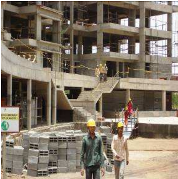
Workforce evacuating the building & moving towards Safe Assembly point
