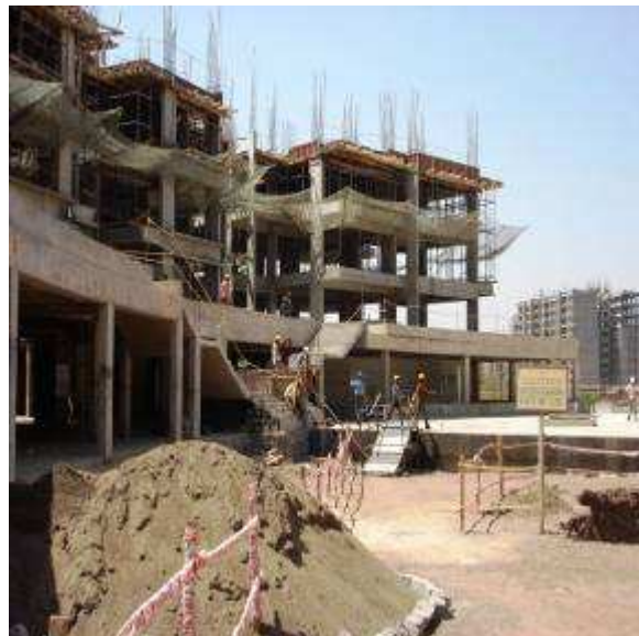
Workers working on the above floors egress through the central staircase towards the safe assembly point- Block II
