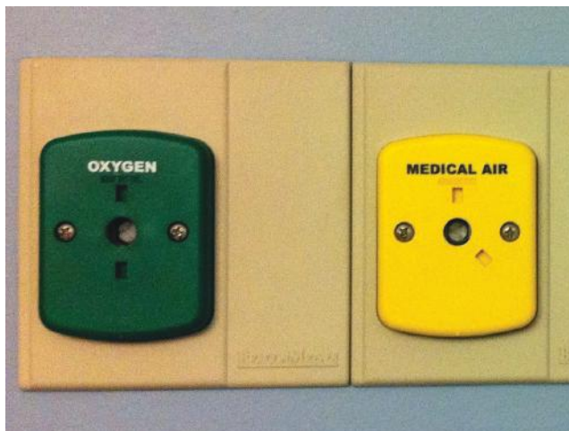
Figure 11.38 Medical gas connectors have good physical error proofing built in.
