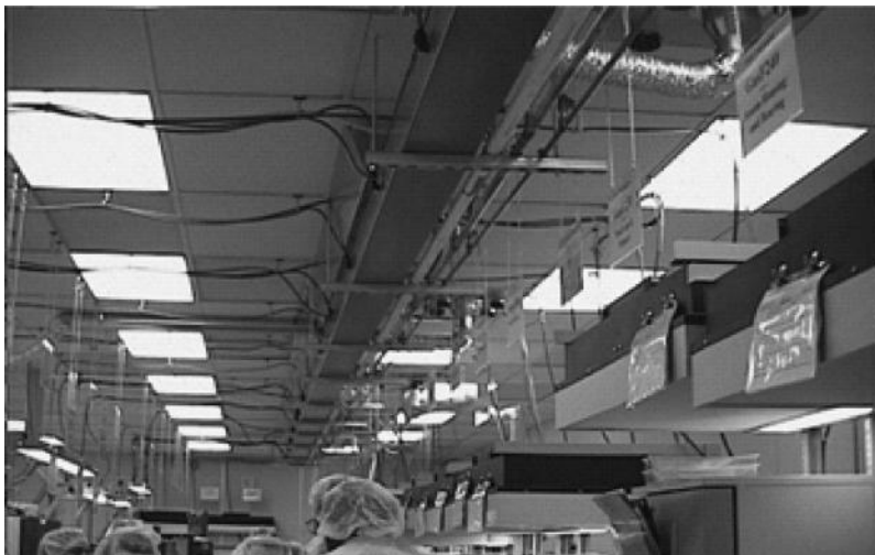
FIGURE 6.15 Flexible Utilities - Clean Room. Source: BIG Archives.
